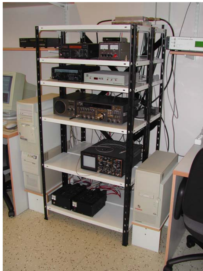
Figure 3. Main inner equipment of the telemetry and command station.
